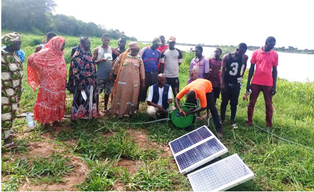
INSTALLING DEMONSTRATION AND TRAINING SITE FOR THE SF2 SOLAR PUMP, MALI (PHOTO CREDIT: EMICOM)
