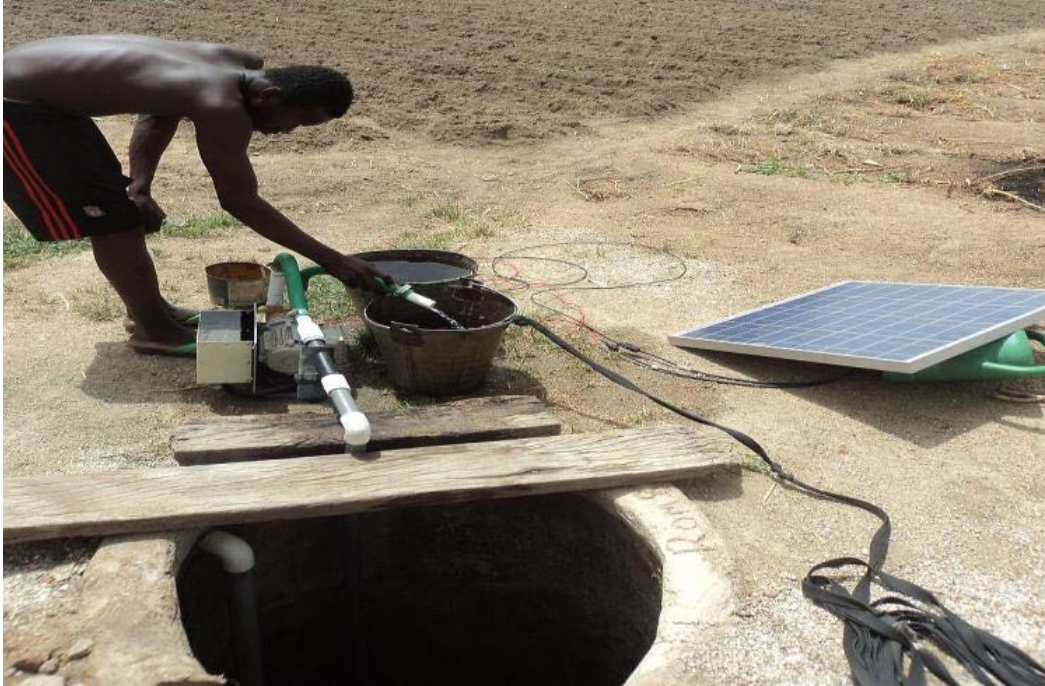
Solar pump installed in Ghana. (Source: Bern University of Applied Sciences, 2013)
