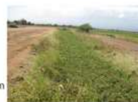
Main irrigation canal (unlined) with poor maintenance
