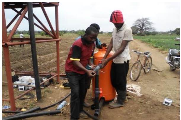
SUA undergraduate irrigation engineering students installing drip systems in Rudewa. Photo credit: SUA
