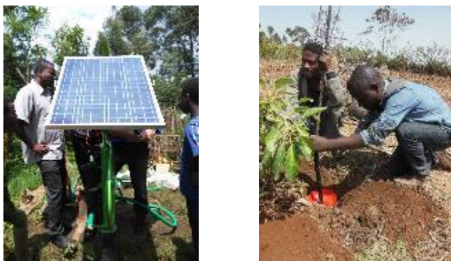
Figure 11: Installation of the solar pump in Upper Ghana together with Practica (left) and installation of wetting front detectors for avocado by the TAMAR students (right).
