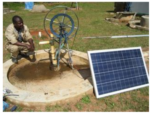
Figure 10: Solar-powered rope-and-washer pump
